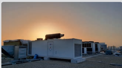
Emergency Power Systems
